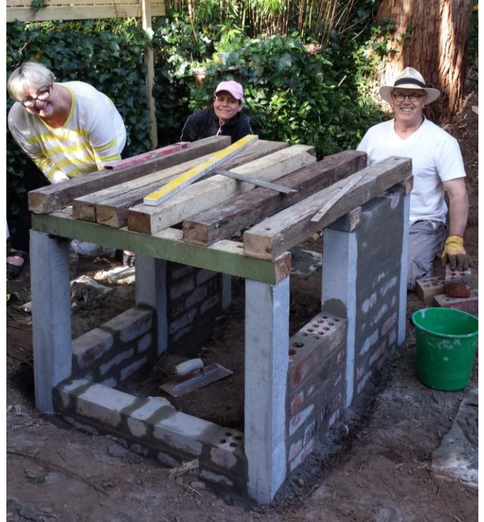
Photograph: Kym Merriman, Nicole Moustakas and Julian Bamford lay bricks to form the walls of the marble Buddha base.
