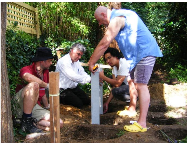
Photograph: Simon Kearney, Frank Carter, Destin Nguyen and Peter Marshall installing the concrete stumps of the marble Buddha base.
