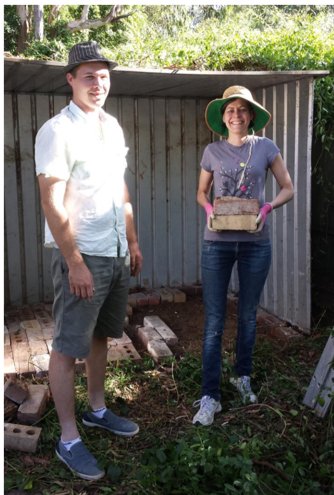
Adam Richards and Nicole Moustakas removing the old garden shed at the end of the driveway in preparation for Anita and Frank's new carport. Photograph by Claire Ransome, 18 th January 2014
